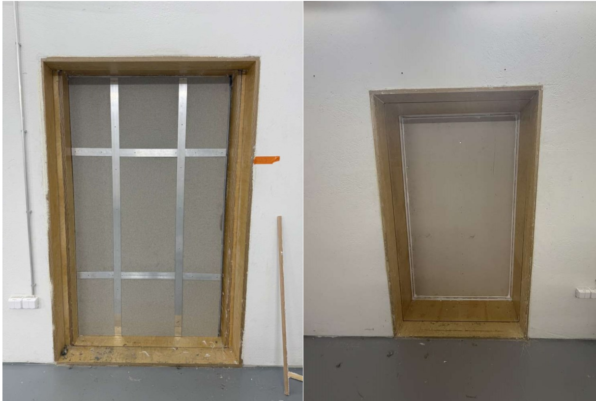
Figure A3.4. The Wall 3 installation into the test opening. The image on the left is viewed from the source room. The image on the right is viewed from the receiving room.).
