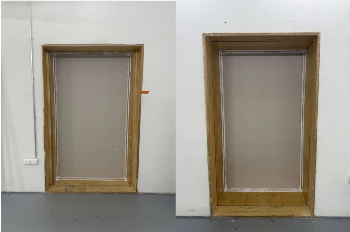
Figure A3.1. Reference wall installation into the test opening. The image on the left is viewed from the source room. The image on the right is viewed from the receiving room.
